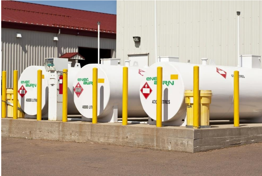
Injection Setup for 100,000 gallon plus fuel tank farm with bulk EnerBurn storage
